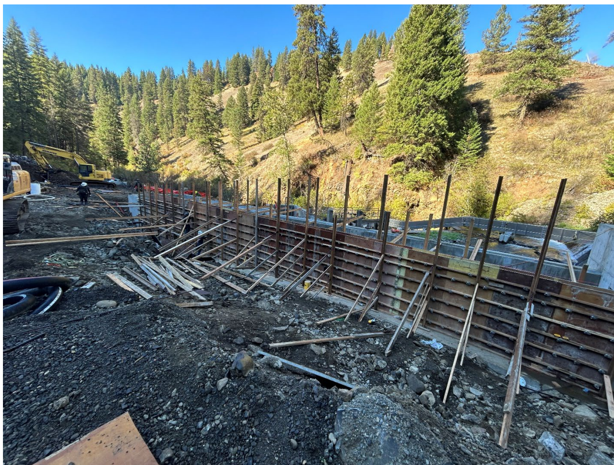
Figure A. Construction of the new fish ladder at Lookingglass Hatchery, October 2025.
